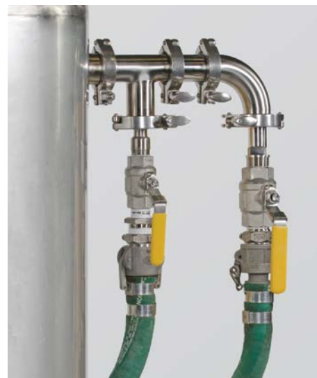
Mixing and injection assembly installed on post-screen piping.
