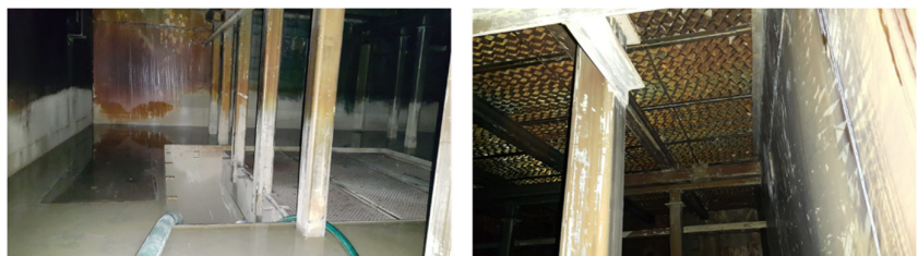
Inspection of condenser after 13 months of sulfur dispersant trial. Note clean surfaces encountered.
