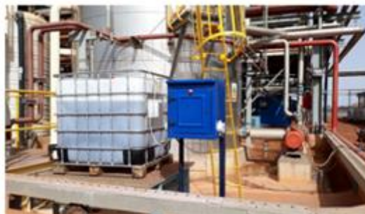
Top – Centralised Dosing System
