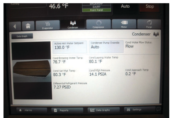
Chiller Approach Temperatures Indicate Heat Transfer Efficiency and Should Be Routinely Monitored.
